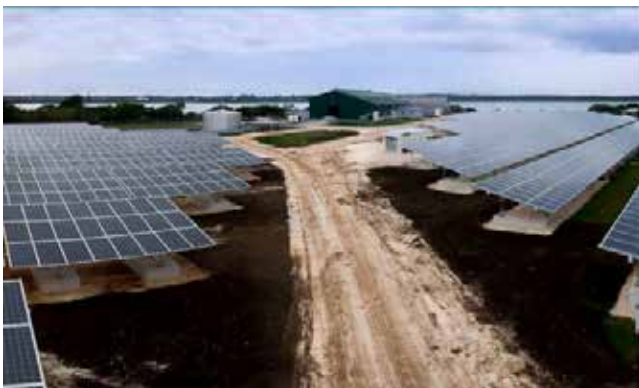
Source: Tonga Power Limited
