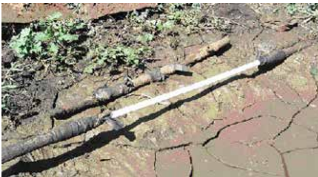
FIGURE 3–12 Leaked pipe repaired with bicycle tubing
