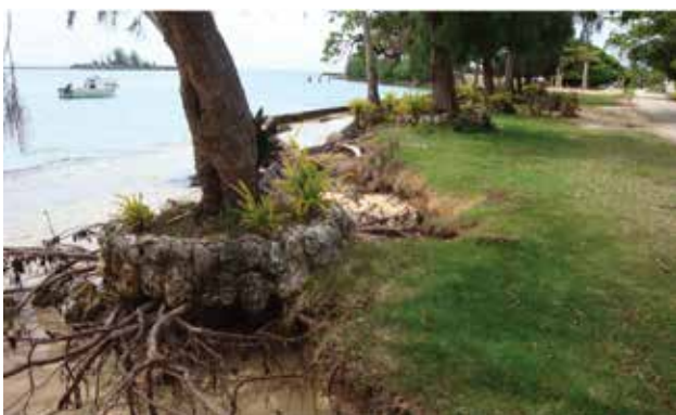
FIGURE 3-44 Erosion at lifuka
