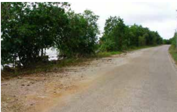
FIGURE 3-43 Over-topping along the eastern part of Tonga
