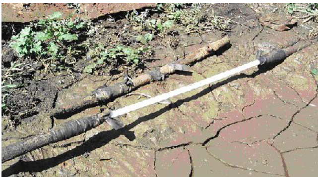
FIGURE 3–12 Leaked pipe repaired with bicycle tubing
