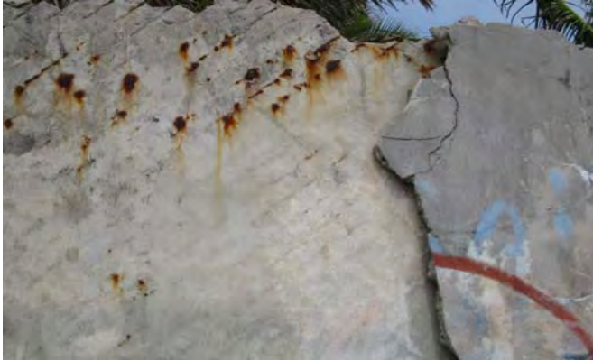
Badly constructed and outdated ferro cement tank.
