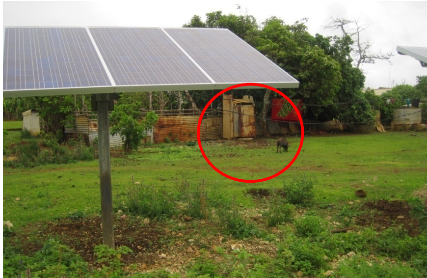
Figure 25: Nomuka, Ha'apai, solar panel that powers pump, with pit latrine and roaming pig in the background (red circle), not more than 30m away. Photo was taking standing next to pump house. (Nicola Fry, 2010)
