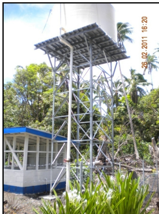
Figure 29: The new well at Kotu Island, Ha’apai, installed in late 2010. The well was producing good water until Cyclone Wilma (27/1/11) washed sea water down the well and made the groundwater salty for a period of time. (MLSNR data, 2011)
