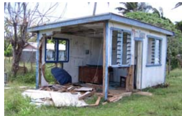
Damage to Ha'apai Meteorological Station by Tropical Cyclone Wilma Jan 2011
